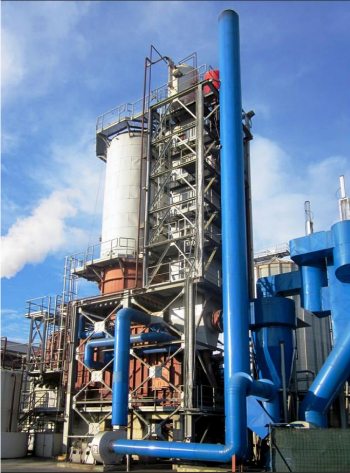
Figure 4-14: Rice husk fueled ORC power plant [16]
