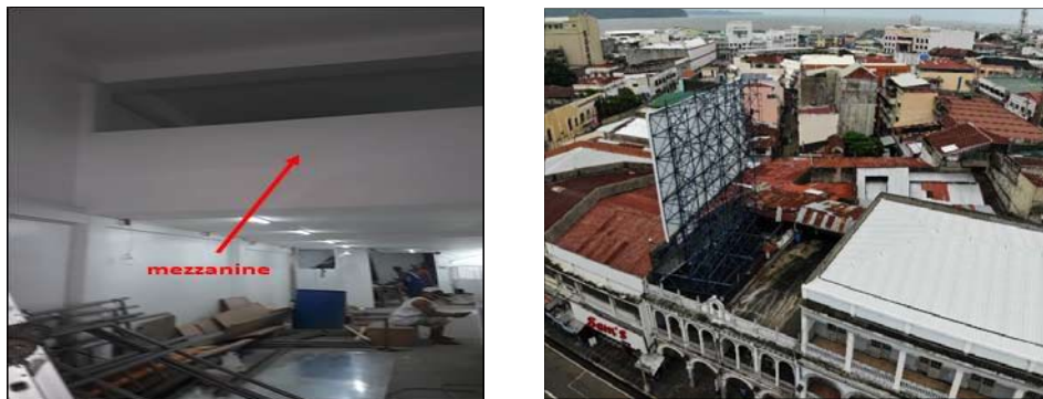
Figure 8. (a) Installation of mezzanine; (b) installation of billboards on top of the structure
